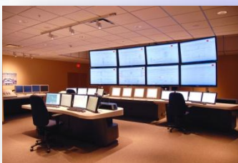
Digital Instrumentation And Control
