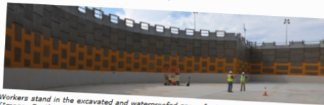
Workers stand in the excavated and waterproofed space for Vogtle 3's reactor building (Image: Southern)
